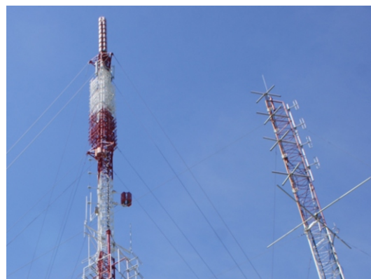
Broadcast towers located in Ciudad Habana. The tower on the left has been identified as primarily a TV broadcast tower, while the tower on the right has a variety of radio equipment.
