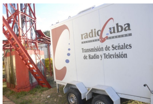
One of Radiocuba's engineering service trailers at the San Isidro Ilegó antenna park south of the city of Sancti Spiritus.
